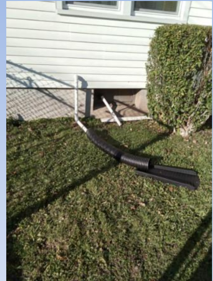
Sump pump discharge to lawn
