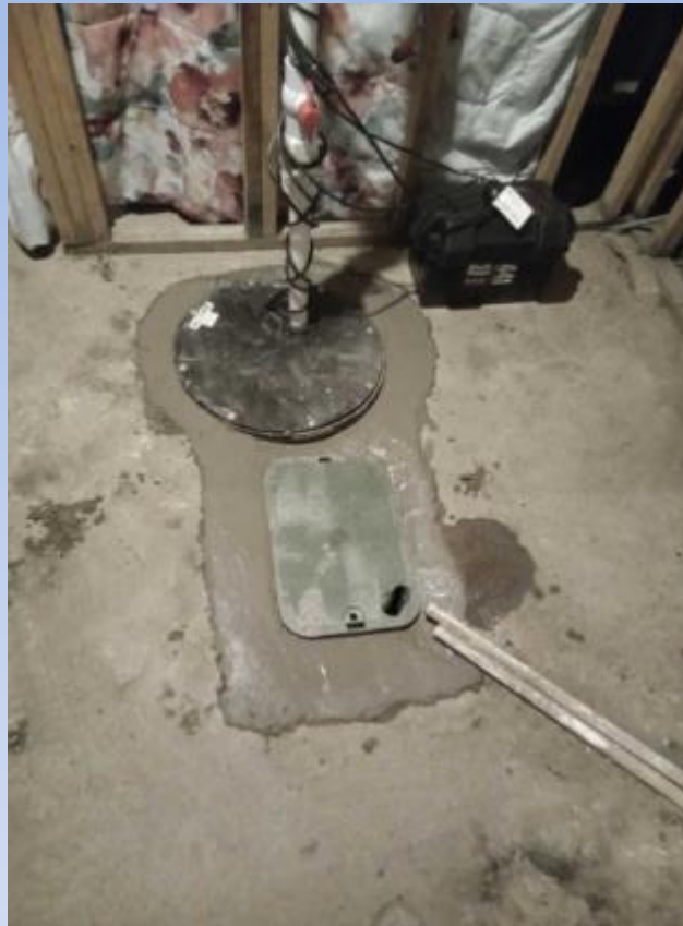
New sump pump (with battery backup) and new Backwater Valve (BWV) inside irrigation style box
