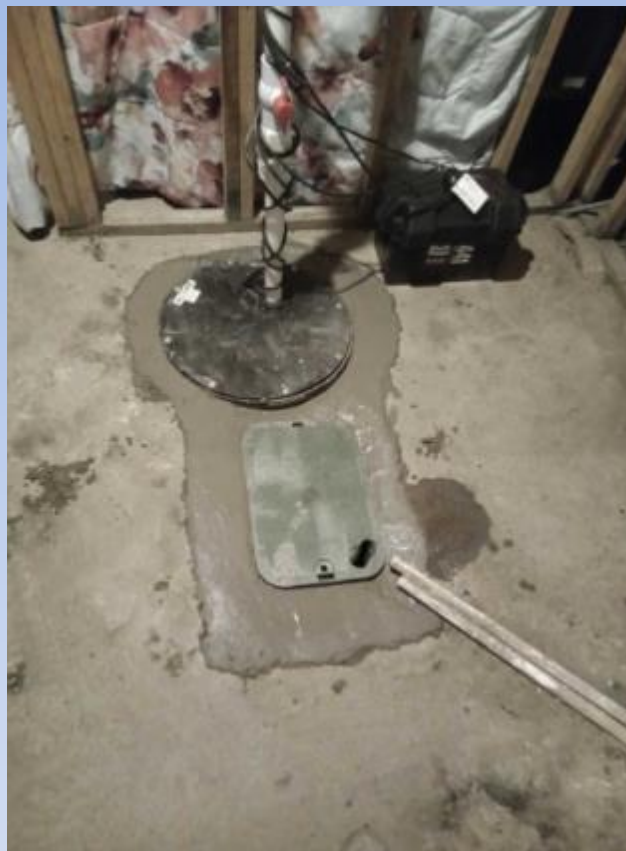
New sump pump (with battery backup) and new Backwater Valve (BWV) inside irrigation style box
