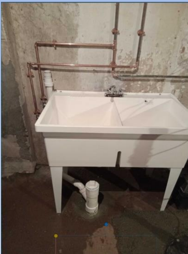
New double bay plastic sink and drain piping (new check valve also installed not in photo)
