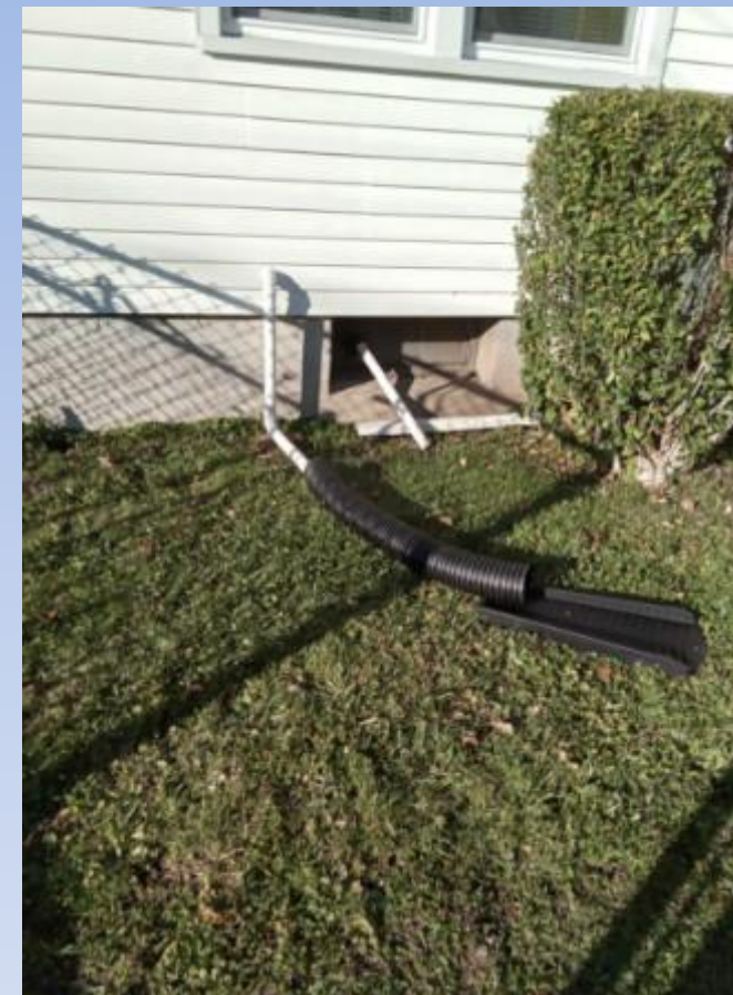
Sump pump discharge to lawn
