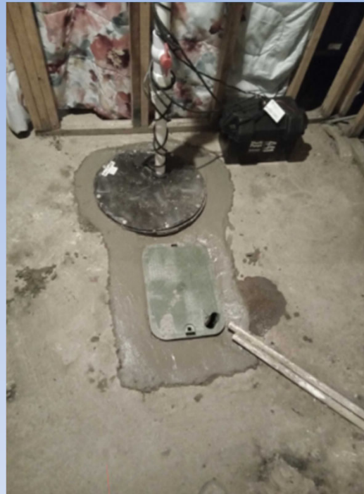
New sump pump (with battery backup) and new BWV inside irrigation style box
