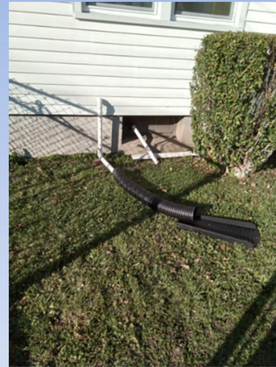
Sump pump discharge to lawn
