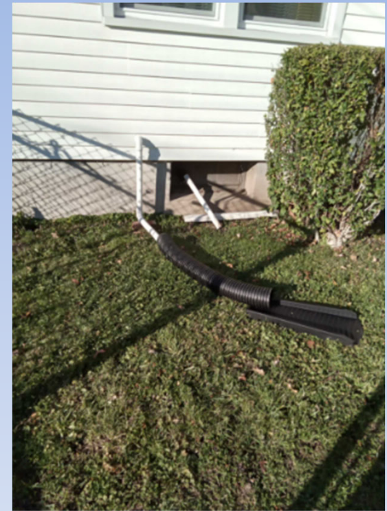
Sump pump discharge to lawn
