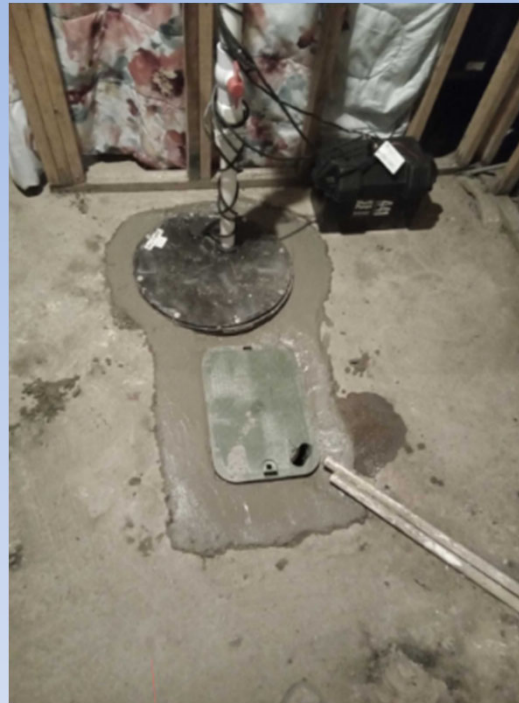
New sump pump (with battery backup) and new BWV inside irrigation style box
