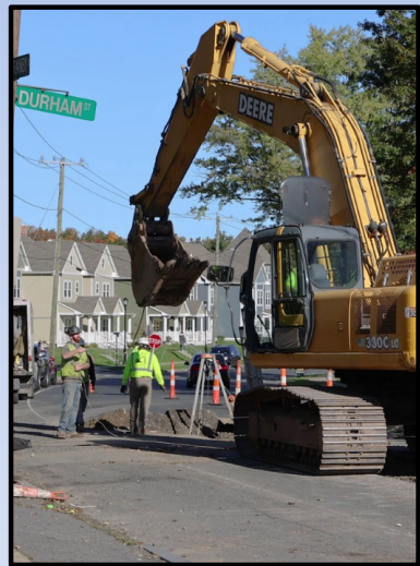
Point repair (Project: Sewer & House Connection Rehabilitation in North Branch Park River Area)
