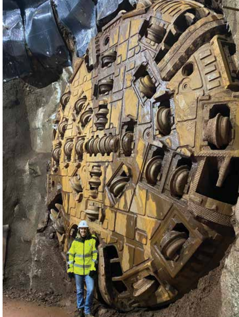
Susan Negrelli, Director of Engineering for the MDC, stands in front of the cutting head of the tunnel borer after it broke through the West Hartford end of the tunnel.
