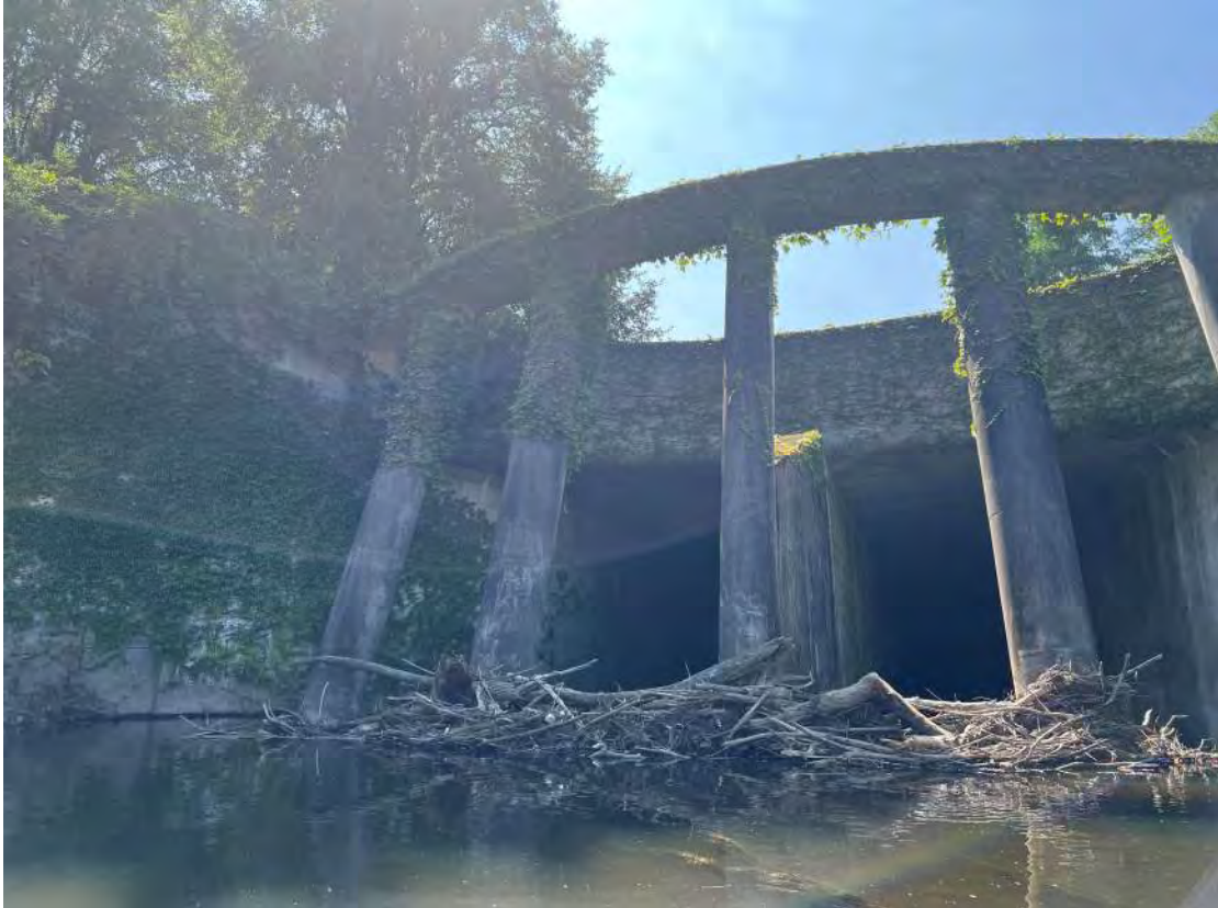
Photo 1: Debris dam at start of Segment 1, Park River Conduit (See Figure 3-1, TD-1).
