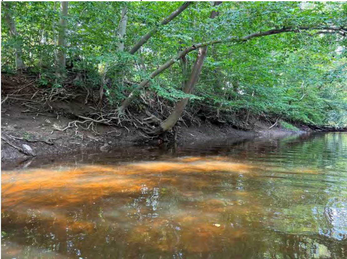
Photo 47: Eroded, steeply sloped banks, undercut trees/roots, bank failure in Segment 4.
