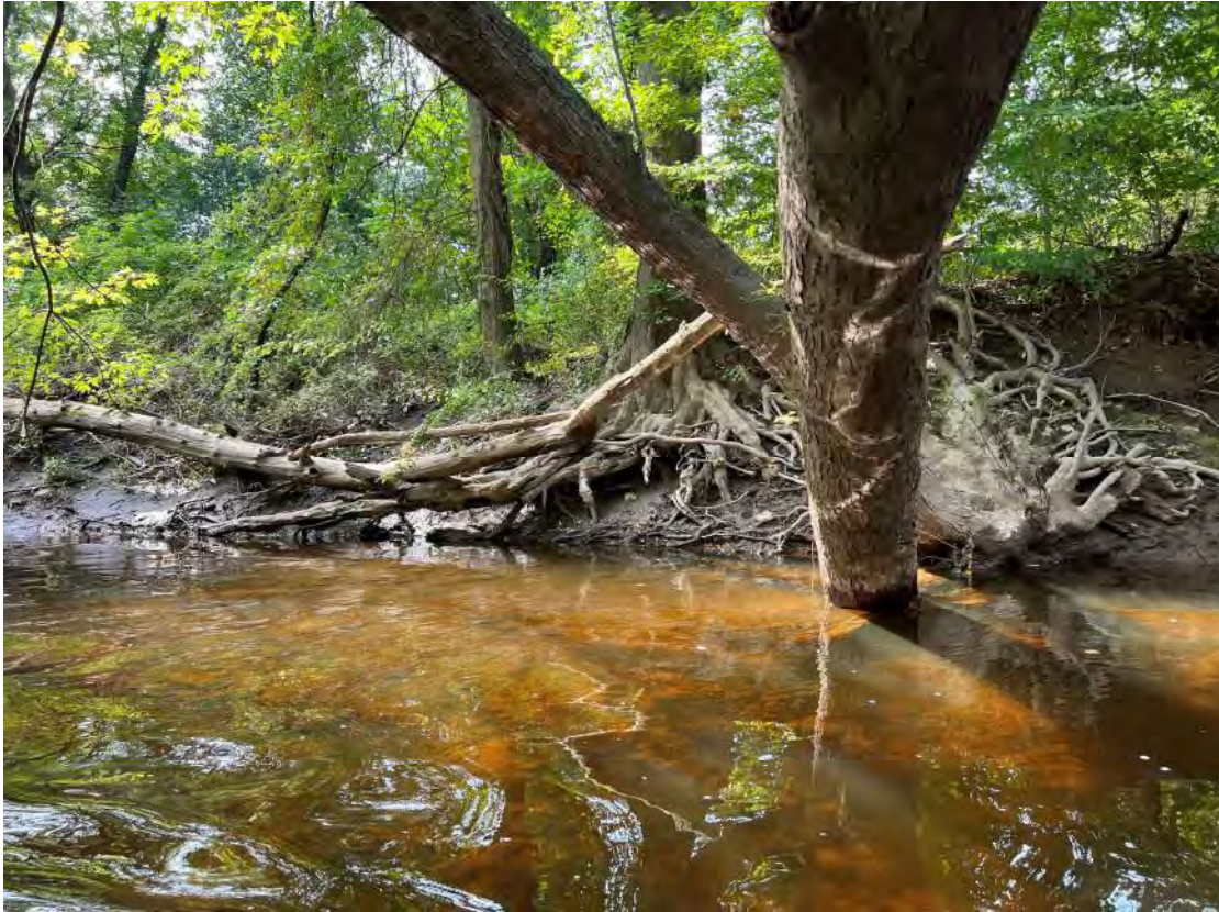
Photo 46: Undercut banks/trees, nearly vertical banks, bank failure, fallen trees in Segment 4 (additional view of trees in area of TD-23).
