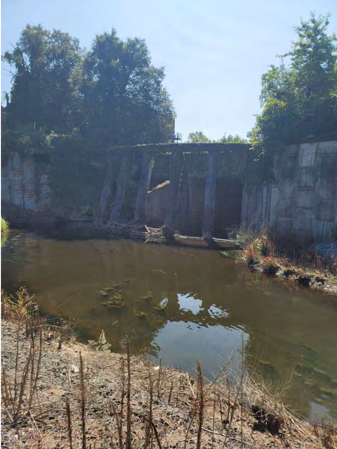
Photo 2: Water pooling directly upstream of Park River Conduit (Segment 1).
