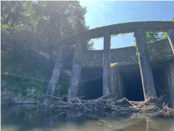
Debris dam at start August 23, 2023
