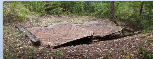
Photo: Rotted Wooden Protective Deck at Weir
