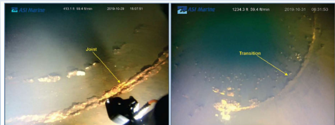
Figure 19: Image of joint at Station 03+41 (left); Image of transition at Station 12+17 (right)
