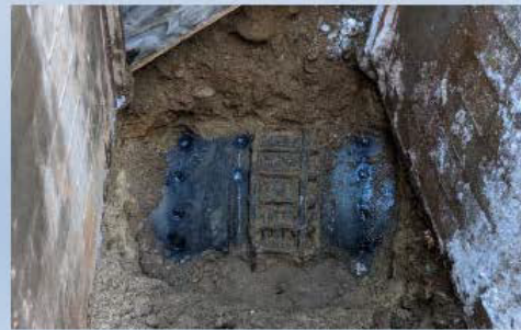
Photo: Exposed Dresser Coupling
