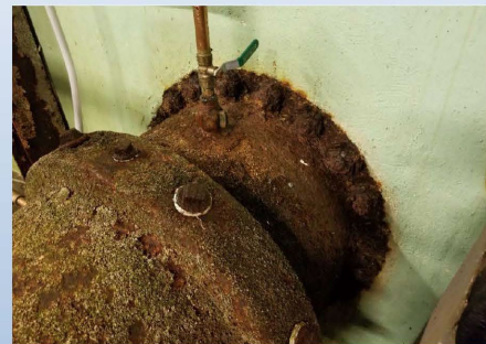
Photo: Corroded Pipe
