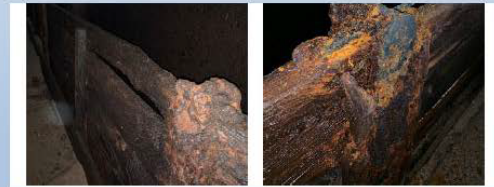
Photos: Baffle deterioration
