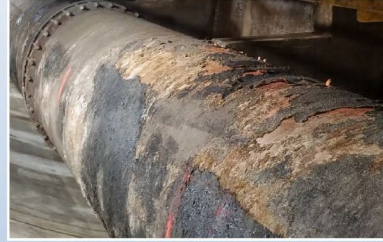
Photo: Damaged Exterior Coating
