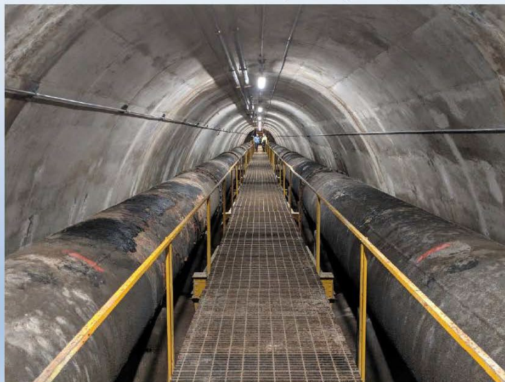
Photo: Steel Mains within Saville Dam Gatehouse
