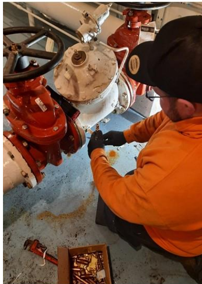
Pressure Reducing Valve - Farmsted SPS
