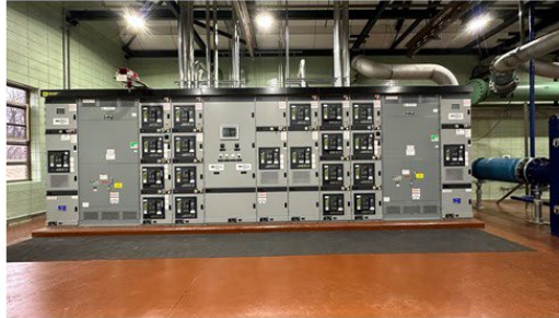
New Main Switchgear
