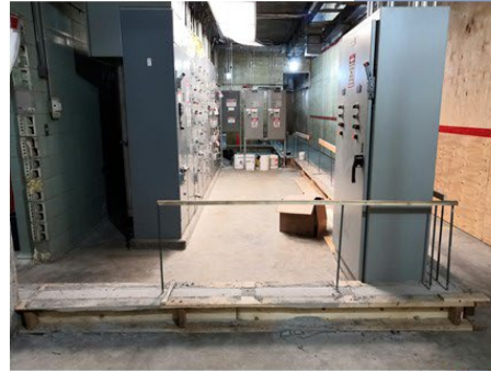
DAFT Electrical Room
