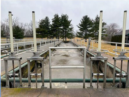
Future Aeration Upgrades
