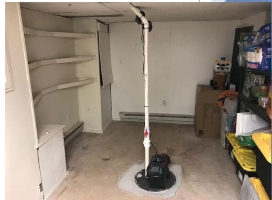
INSTALLED SUMP PUMP WITH BATTERY BACK UP
