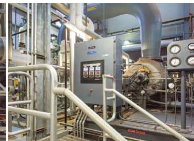
Hartford’s Steam Turbine—the steam then spins a turbine that is connected to a generator and produces electricity that directly offsets HWPCF’s power costs
