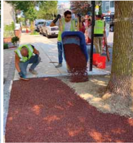
Porous flexipave increases water retention
