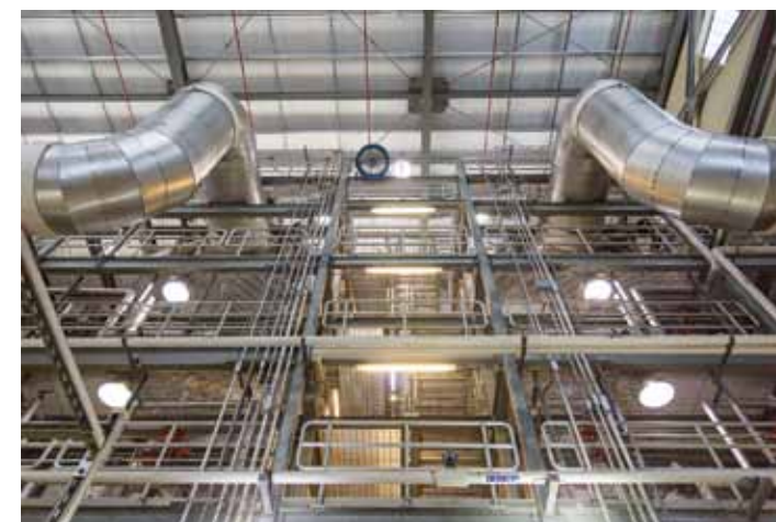
Ground level view of Hartford’s two heat recovery boilers—the HRF takes heat from the incinerator exhaust and turns it into steam in large boilers
